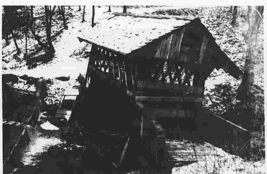
The covered bridge across Porter Brook in the Oak Grove Nature Center was to be torn down Saturday. The bridge has been closed for about a month because it has structural problems and is considered a safety hazard. Patriot Lane resident Alex H. Krajevski is organizing a drive to save the bridge.
